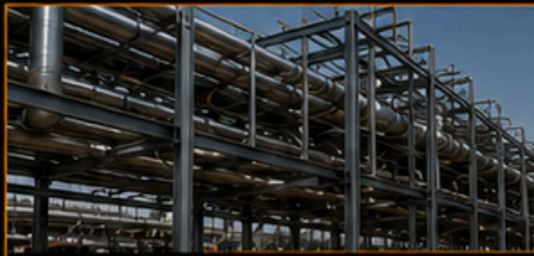
PIPE RACKS & SUPPORTS
